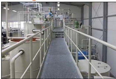
A FENTOX plant in the chemical industry
