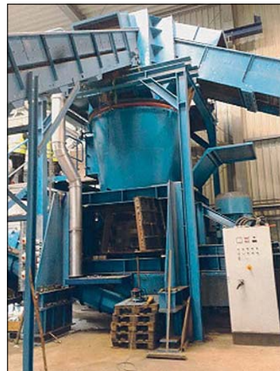
CompoCycle – fibreglass recycling plant
